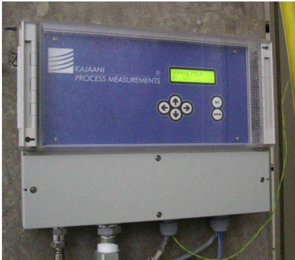
Figure 3: Local control box
